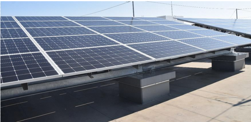
Yokohama Kankyo Design's solar PV panel mount (SUSK) is installed using a roof-top renting scheme (site: Shoko High School, capacity: 57kW)
